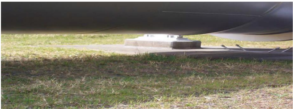
Figure H.4 – Typical Warragamba pipeline arrangement near plinth, estimated gap 0.3m (Photo source tenders.nsw.gov.au)
