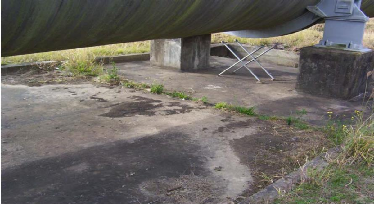
Figure H.3 – Typical Warragamba pipeline arrangement near plinth, estimated gap 0.5m (Photo source tenders.nsw.gov.au)
