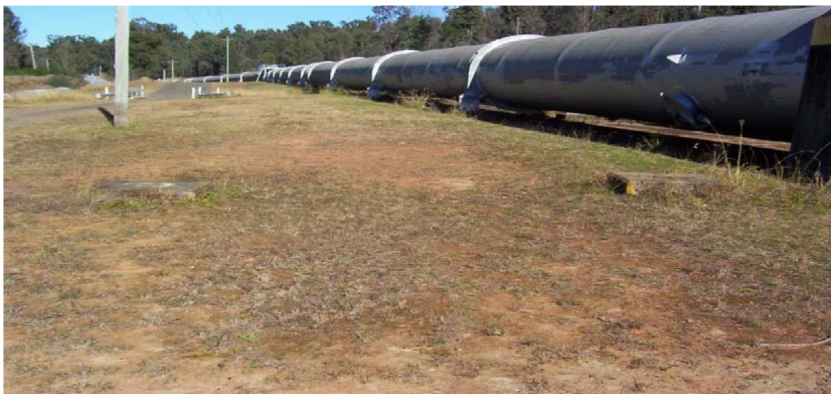
Figure H.2 – Typical Warragamba pipeline arrangement (Photo source tenders.nsw.gov.au )
